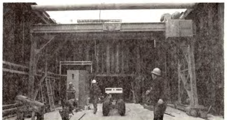
...Construction of the P-Central experimental pit. Light-colored box at rear center contains target box...
