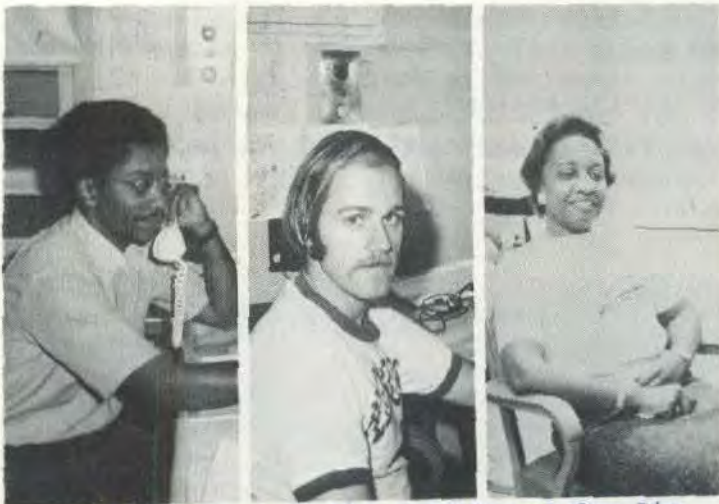
...Last few days on the cord board for Jim Lasenby, Bill Marquardt, and Jean Van Lear. The NAL switchboard has been located at 22 Potawatomi since 1968. The switchover to Centrex will be complete on Monday, November 6th. Employees should notify frequent callers of the change...
