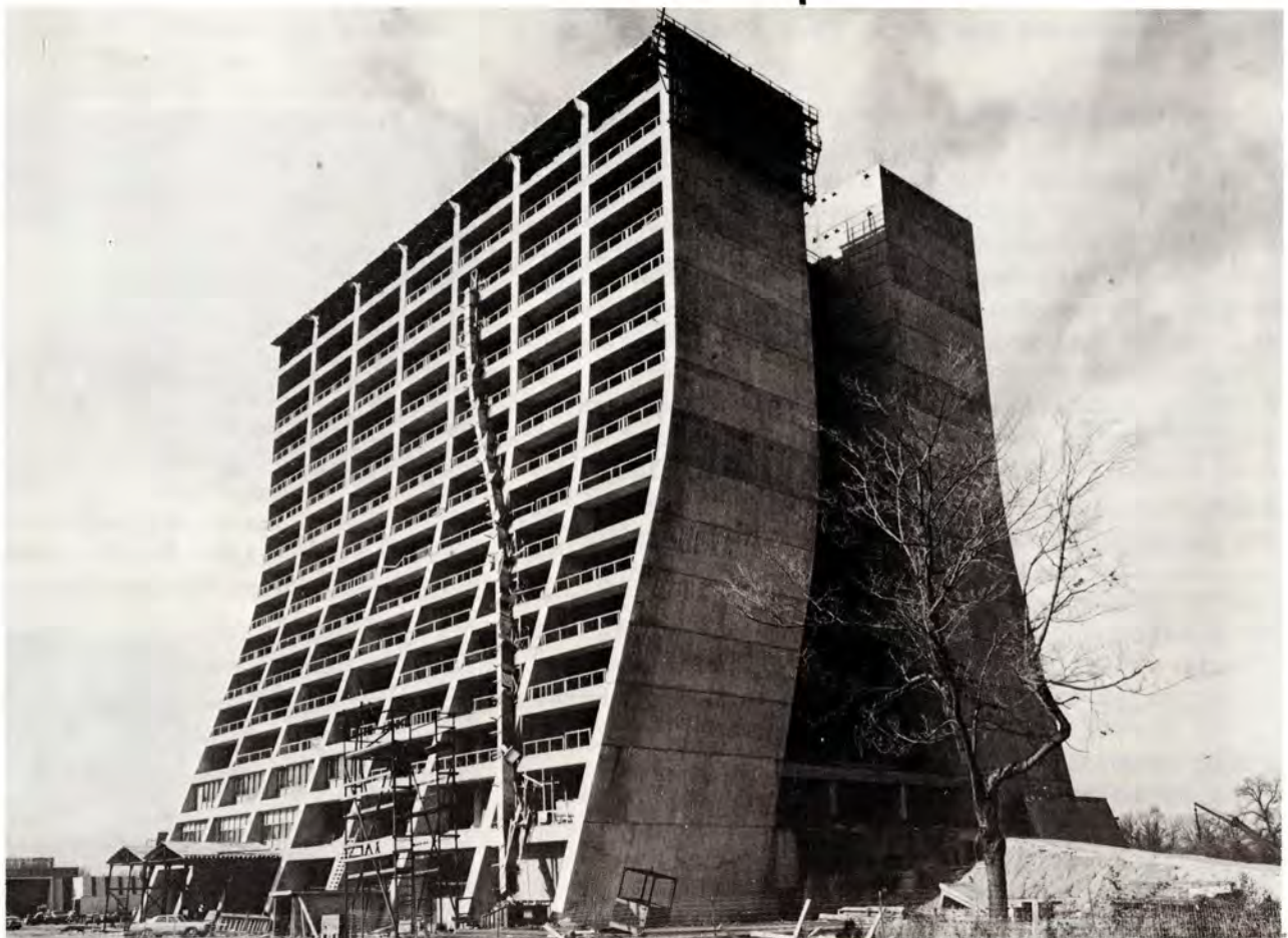
...The top floor of NAL's Central Laboratory Building is now being poured. The building will be ready for occupancy some time after March, 1973. It will house many of the functions of the Laboratory including all of those now located in the NAL Village...
