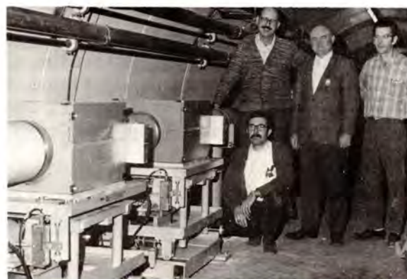
...Involved in the installation of the beam scraper were (kneeling): R. Ducar, Accelerator Section; standing L-R, H. Barber and L. Bradstreet, Technical Service; W. Martin, Accelerator section...
