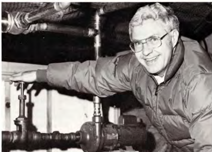
...John O'Meara, president of Solar Energy Club, opens valve to start flow of solar heated water at Fermilab...
