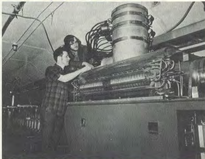
....Rich Howel, top, and Fred Sarver, standing, install magnet shields in RF unit in Booster tunnel....
