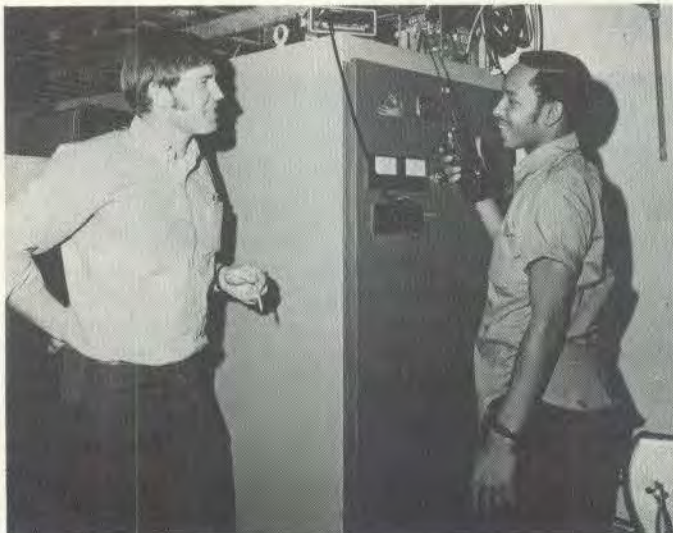
....Rich Janes and Ed Stitts read power supply monitor for septum magnet being tested below in Booster tunnel....
