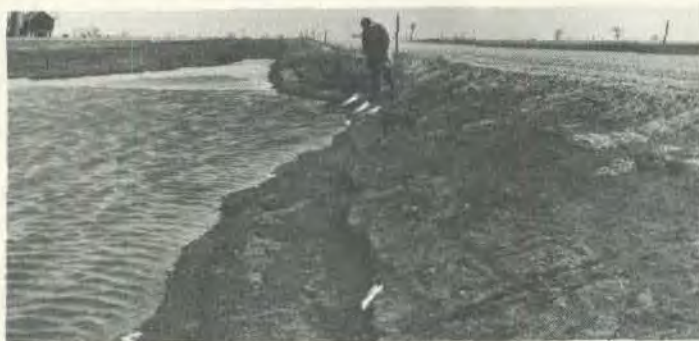
....A one-day accumulation of water, some 2½ feet deep, pumped from one of the low spots on NAL site....
