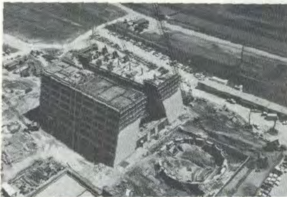
...A recent aerial photo of the construction progress on the NAL high rise-auditorium complex...
