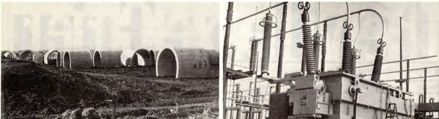
...Main Ring and Master Substation, two of DUSAF's many challenges in six years at FermiLab...
