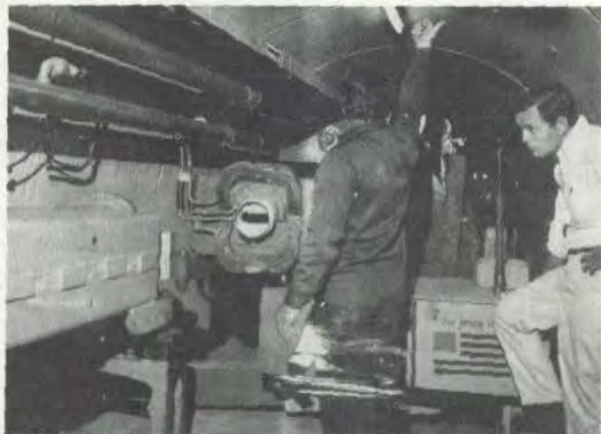
...(L to R) Tony Winchester, George Hill install a replacement magnet in the Main Ring Tunnel...
