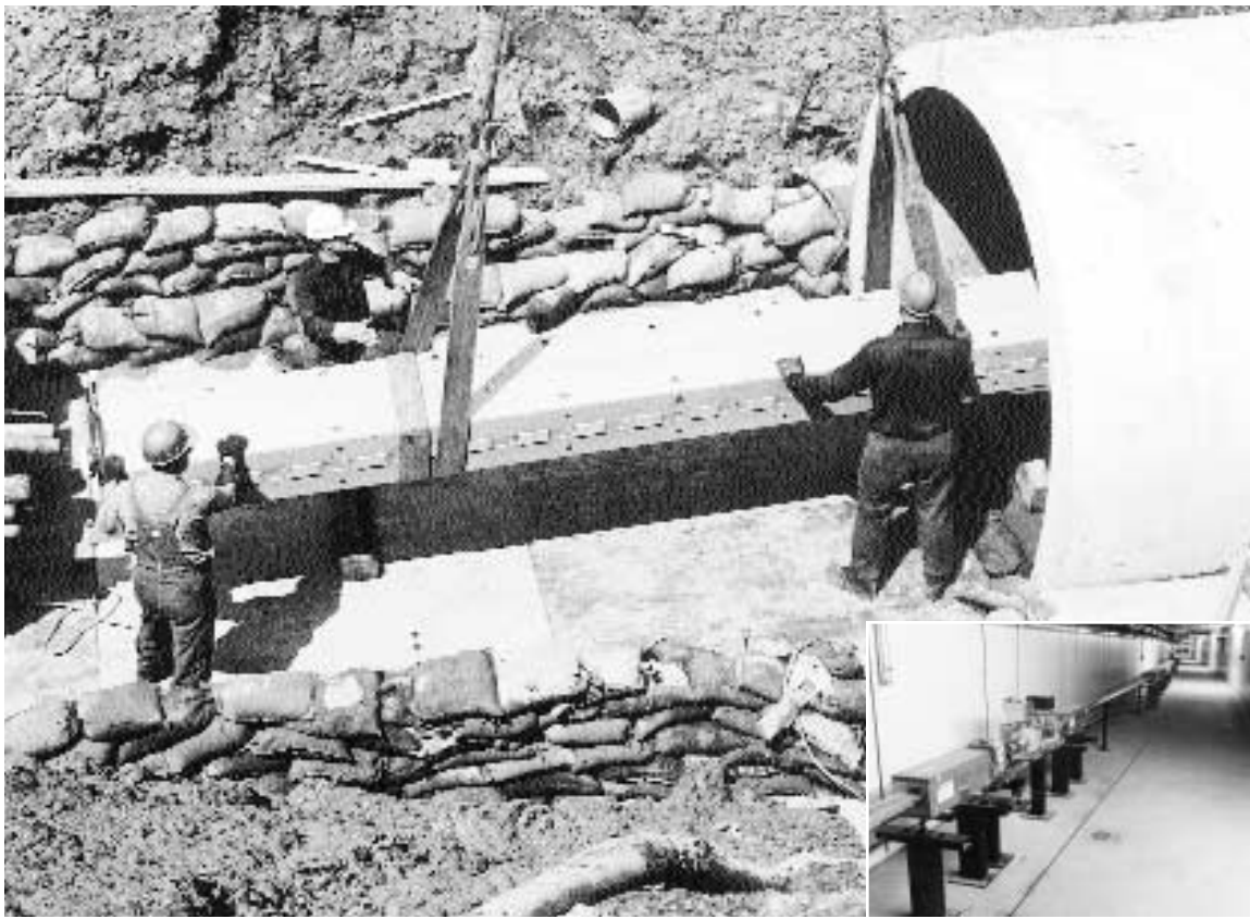
Construction of the Main Ring, with the first magnet set in place, in April 1970. Inset: Fermilab's spanking new 8-GeV beamline.
