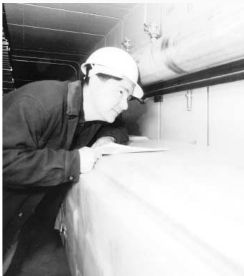
Patrick Hurh inspects one of the 4,000 welds that were repaired in the LCW system.
