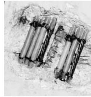
Post-tensioning cables originally were sheathed in hard plastic and encased in the concrete beams.
