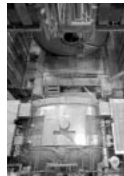
The Lab is focused on completing the detector upgrades to DZero (above) and CDF (below). Craig LeRette and Ron Olsen install wires in the CDF end plugs.
