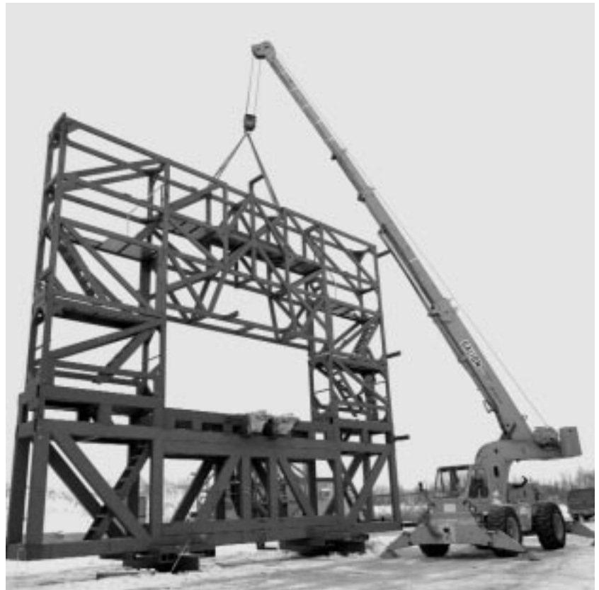
Outside Lab F, a crane truck assembles the truss from its four components, with two smaller sidepieces and a top frame added to the 25-ton base unit.
