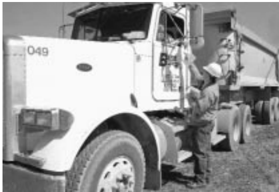
The first of a months-long parade of trucks arrives at the NuMI construction site.
