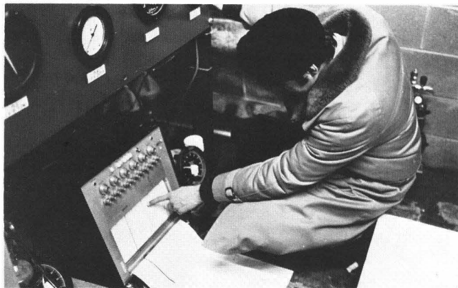
...C. Rode at A-1 refrigeration building during test...
