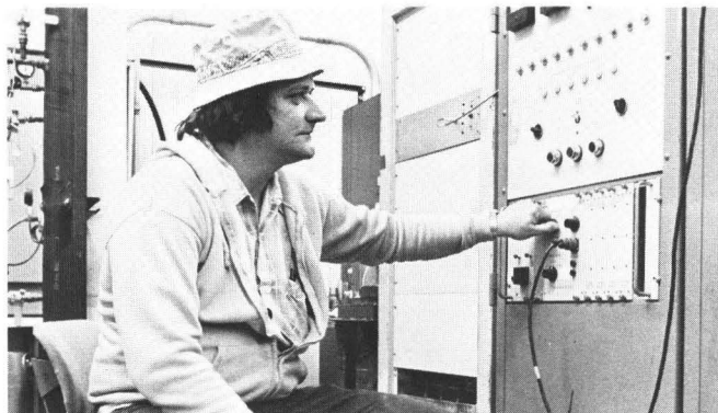
...Bob "Obie" Oberholtzer at Switchyard controls...
