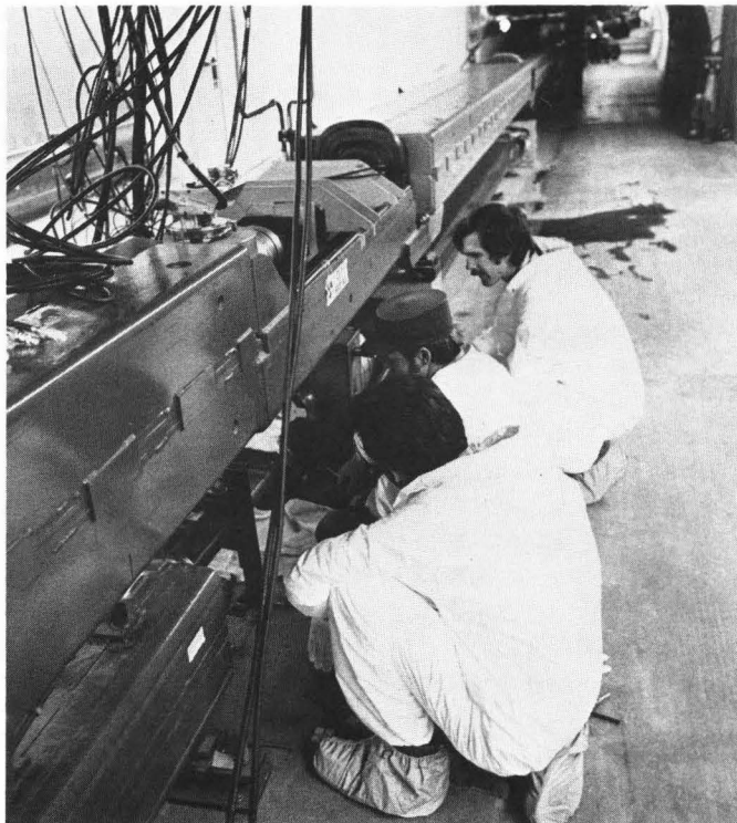
...Installing shielding around beam position monitor are, from left, R. Bennett, J. Smith and T. Peterson...
