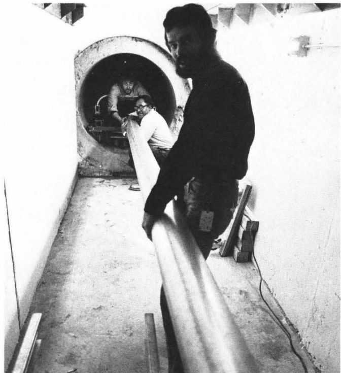
...Installing a section of vacuum pipe in the Meson Target Hall are, (L-R), Bob Jensen, John Williams and Pat Liston...
