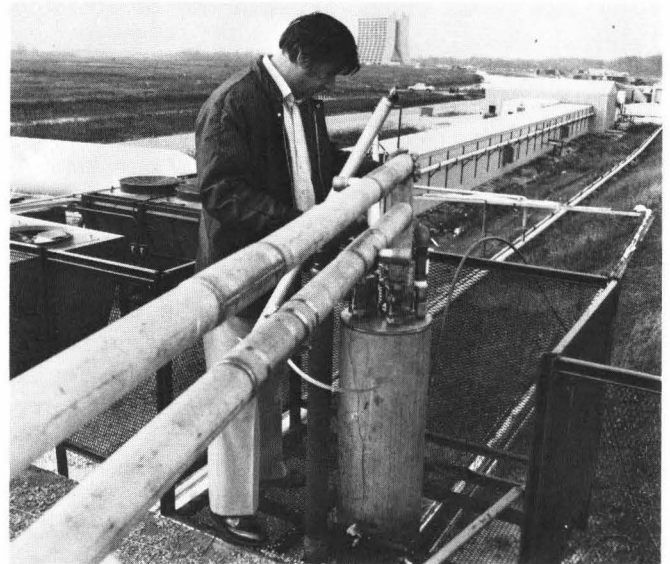
...Karl Koepke examines the connection box to the helium transfer line that runs between the B-1 satellite refrigerator and the B-12 test area, the long building in the background...
