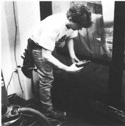
Storm window installation was completed in April and is estimated to save the Lab $139,044 in heating and cooling costs during the first year.
