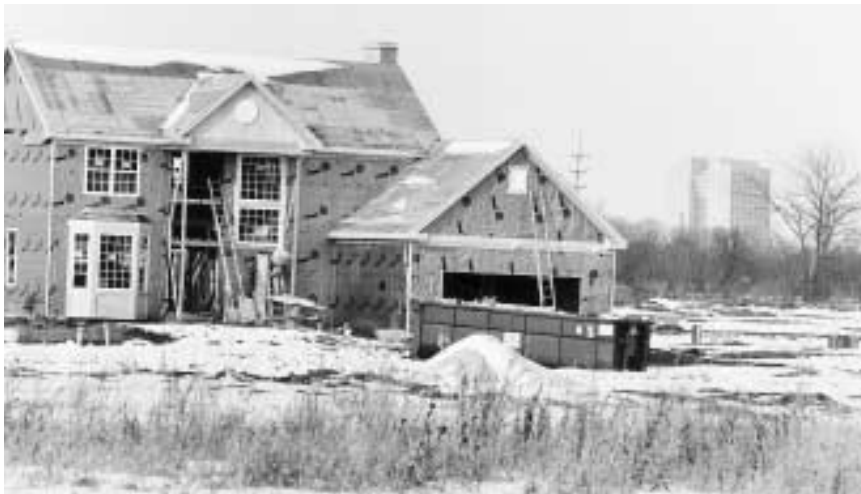
A house being built in Batavia. Fermilab's Wilson Hall rises in the background.
