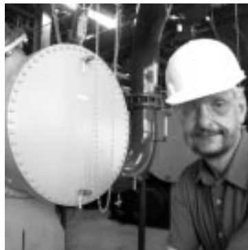
Steve Krstulovich, of FESS, said "Every cooling system at Fermilab was operating at or beyond its design capacity!"
