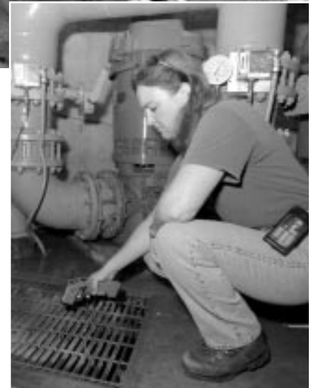
Fermilab maintenance planner Susan Sprosty checks the temperature in Casey's Pond, aiming an electronic thermometer at the water lapping a few inches below a grate in the pump house floor. Water temperature reached 84 degrees, close to the point where it ceases to cool.
