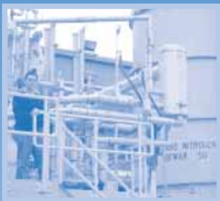
The CHL facility features a complex system of pipes and valves. Mike Geynisman knows their functions inside out.
